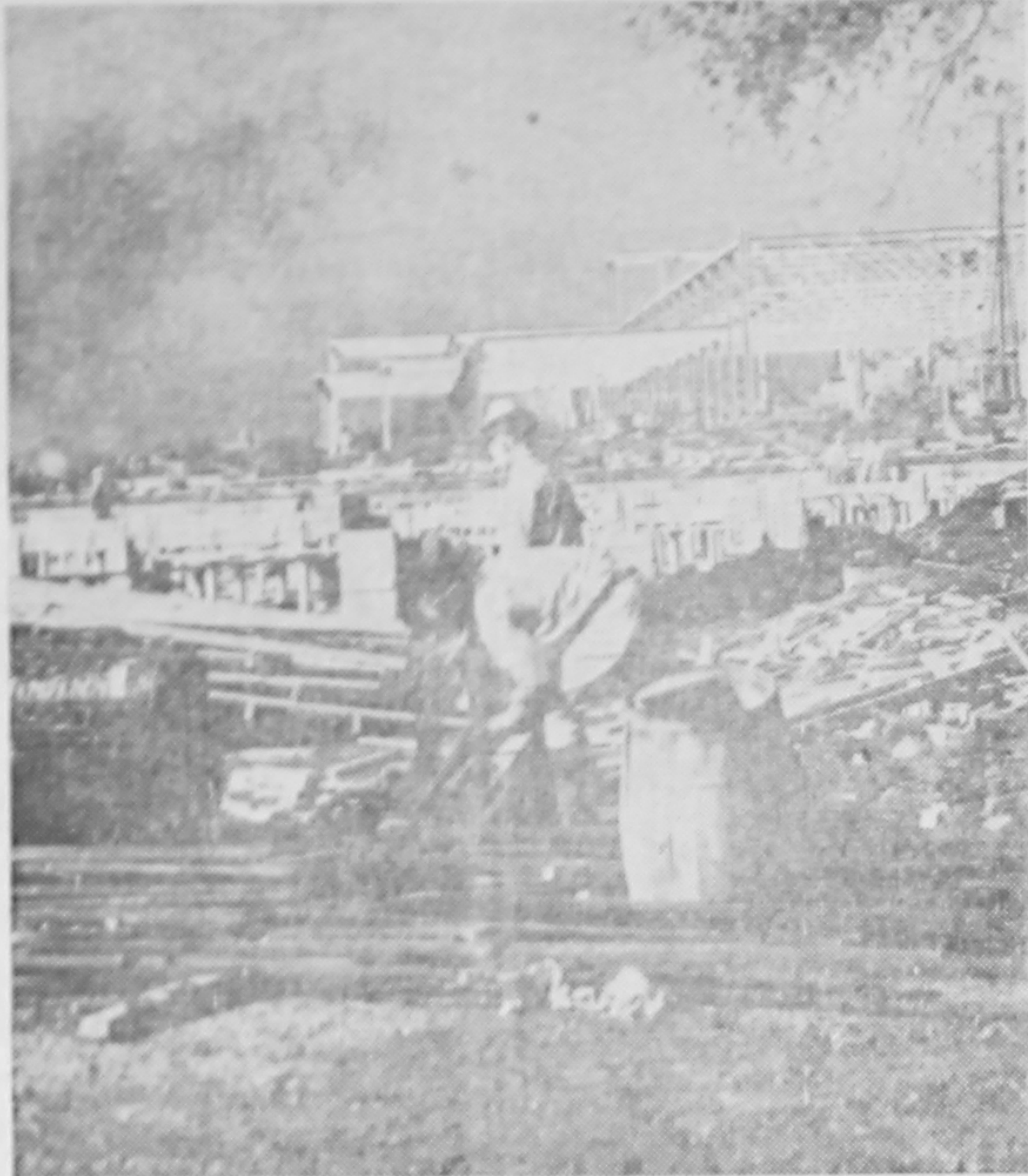
The steel frame of the $140,000 Livestock Building No. 2 for the Texas Centennial Exposition at Dallas can be seen above as it rapidly takes form. With the $260,000 Livestock Building
