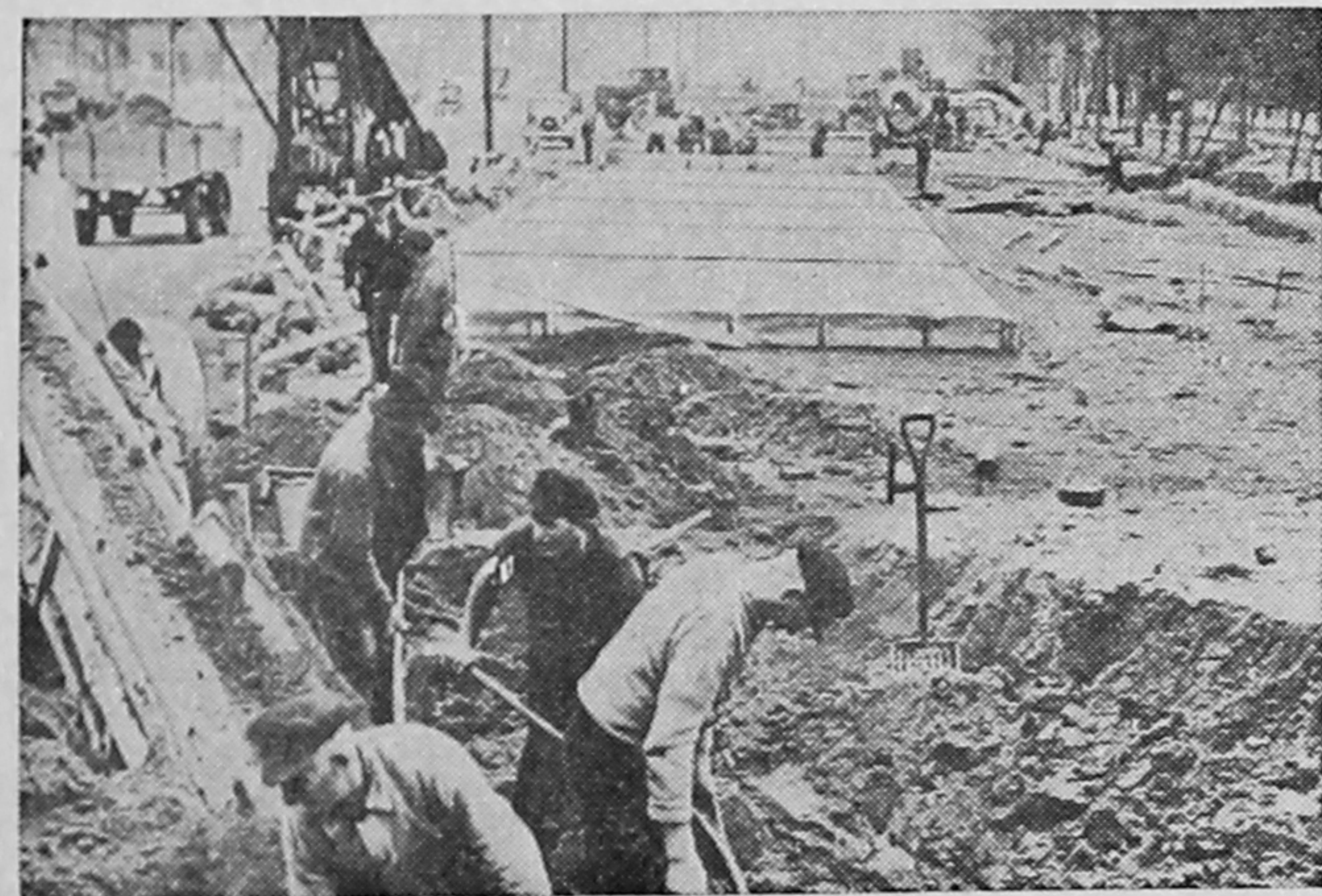
Construction work goes rapidly on the new broad highway that will bisect Berlin from west to east and is a part of the vast road-building program undertaken by Hitler. In 1938 a total of 1,864 miles were added to the country's system of express motor highways.
